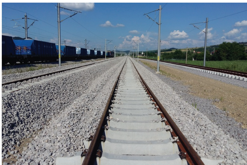
Rehabilitation of the railway line Brasov – Simeria, component part of the IVth Corridor for the train speed of maximum of 160 Km/h, section Coslariu – Sighisoara, Romania Source: National Railway Company „CFR” SA”
